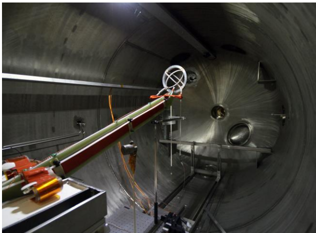
Figure 22. Magnetoshell installed in chamber. Shown are two in-chamber power supplies (potted), low-inductance stripline, G-10 mount.
