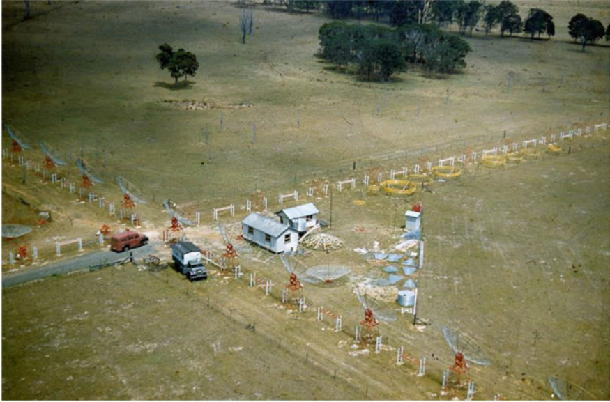
Fig. 4.16 An aerial view of construction work on the Chris Cross in November 1956 showing the construction huts near the centre of the array, some completed aerials and the hooped steel for producing more aerials (CSIRO Radio Astronomy Historical Photographic Archives P10329-6)
