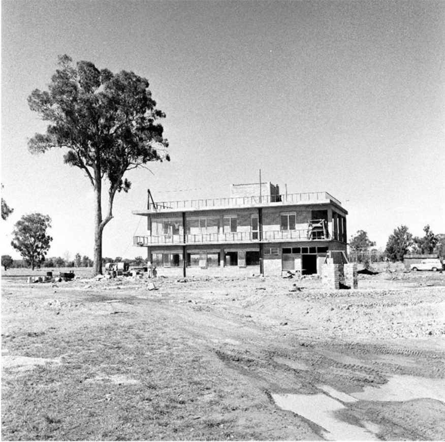
Fig. 5.30 Construction of the receiver and computer building at Culgoora in 1964 (CSIRO Radio Astronomy Historical Photographic Archives B7660-5)
