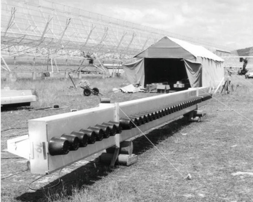
Fig. 3.26 The construction of MOST. The 408 MHz dipoles were replaced with 7744 ring elements that were phased by differential rotation under computer control to track a field for 12 h. Black flower pots were a novel way of protecting the ring antennas. In the MOST configuration, only the east-west arm (visible in the background) of the original cross was used (Courtesy of the University of Sydney Archives)
