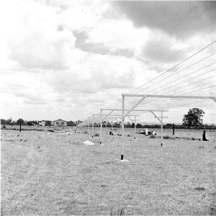
Fig. 3.9 Construction of the east-west arm of the 85.5 MHz Mills Cross at Fleurs field station in October 1953. The view is looking west with the base of the array arm mesh “chicken wire” reflector support frame in place. The receiver hut is visible in the background (CSIRO Radio Astronomy Historical Photographic Archives 3174-25)
