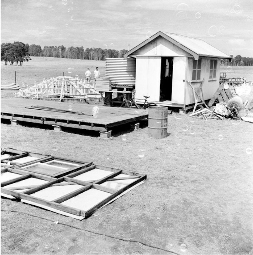
Fig. 4.15 Construction of the Chris Cross underway at Fleurs field station October 1956. This small hut near the centre of the array was used to assemble the components of the cross. To the left of the hut is the aerial frame jig (CSIRO Radio Astronomy Historical Photographic Archives B5006-7)
