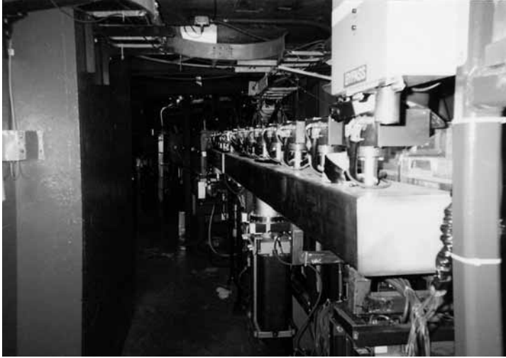
A section of the tunnel in 2001, showing the synchrotron as it bypassed the particle physics detector. (P. Doing)
