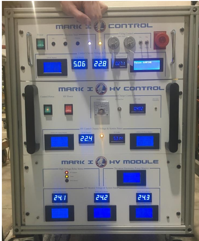
Figure 5. Control panel for portable DPF. LED indicators provide user feedback on control system status, 2-key system ensures that DPF cannot be charged accidentally, and emergency stop de-energizes capacitors through dump resistors in an off-normal event.
