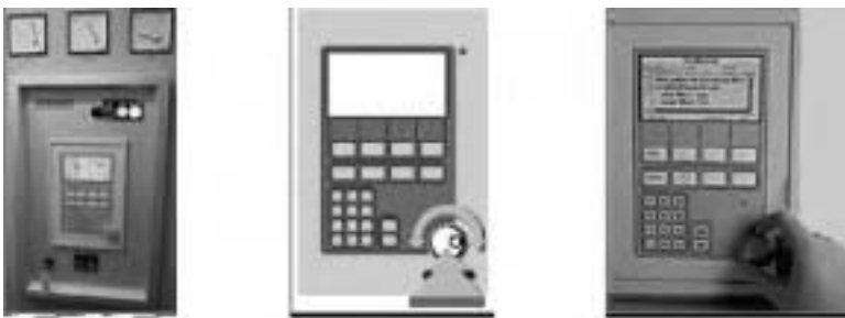
Fig. 14.19 Example of a command panel (left) with user interface 'turn and push' (centre) and human interface with PLC (right) of a microwave plant.
